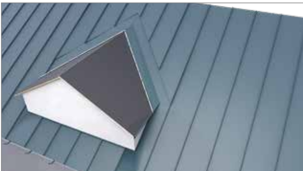
Continue in the same way around the entire ridge. Sheets that touch the wall of the ridge should have a fold of 25 mm.
