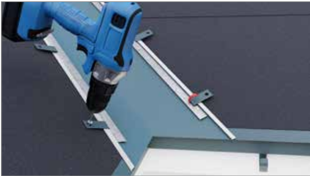
Fold the fastening sill over the edge and fasten with screws. These will be the valley channel's fixing points in the roof.
