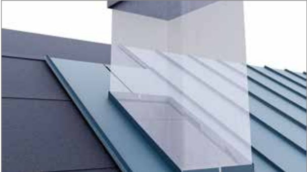
Cut out the sheets for the chimney. Leave 50 mm for folding around the chimney. Cut away the joint above the chimney so you get a level surface.
