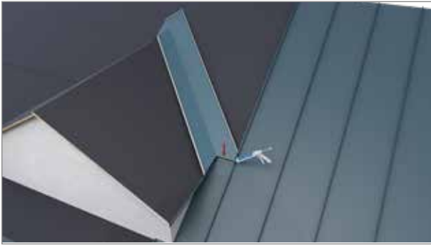
Lay a string of sealant at the top to prevent water penetrating between eaves board and valley.
